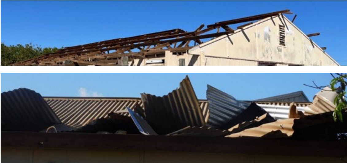
Roof damage to older buildings
