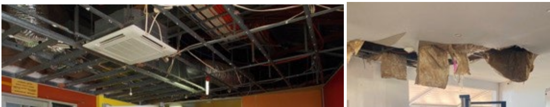
Ceiling loss under a vent in the roof space
