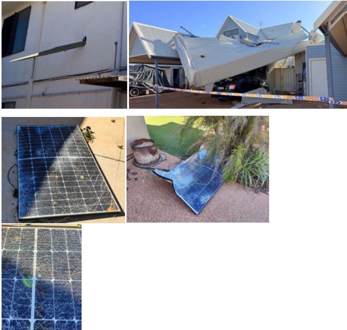
Windborne debris in Exmouth, piece of timber, section of complete roof, solar panels
