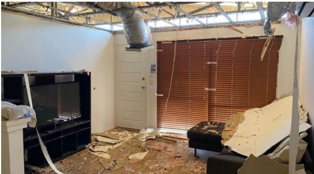
Ceiling loss following damage to a veranda
