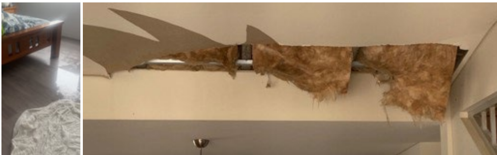
Rainwater passing up a roof slope, water falling from the top of a valley gutter and ceiling loss under a box gutter
