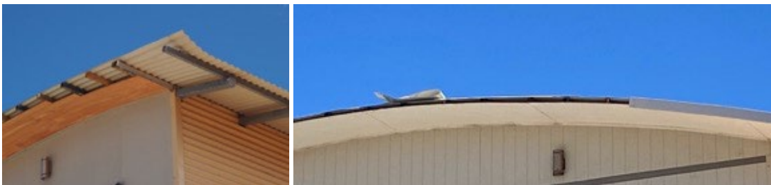
Damage to a flashing that caused ceiling loss inside the building
