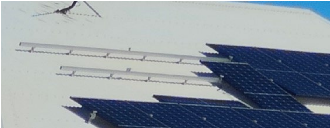
Clamp failures allowed panels to move on the roof and be blown off the roof
