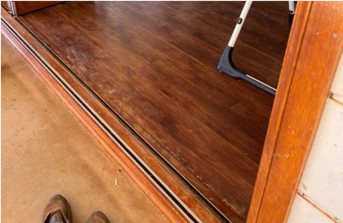
Significant volumes of water came under this bifold door as there was no seal
