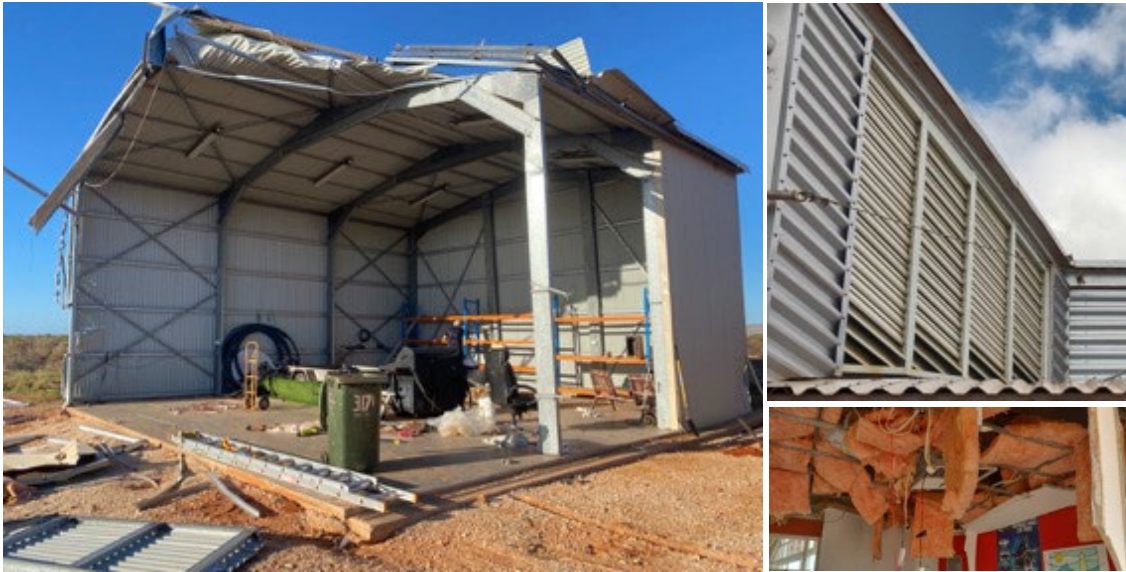
Damage following internal pressure
