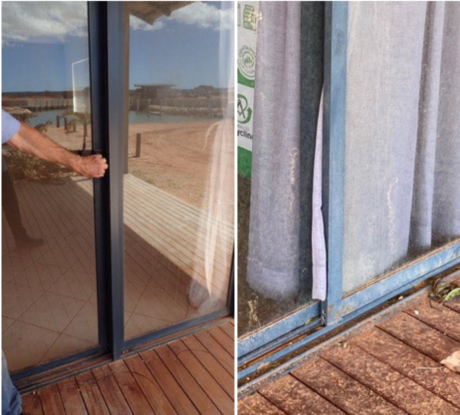
Bowing of lightweight sliding door causing water entry
