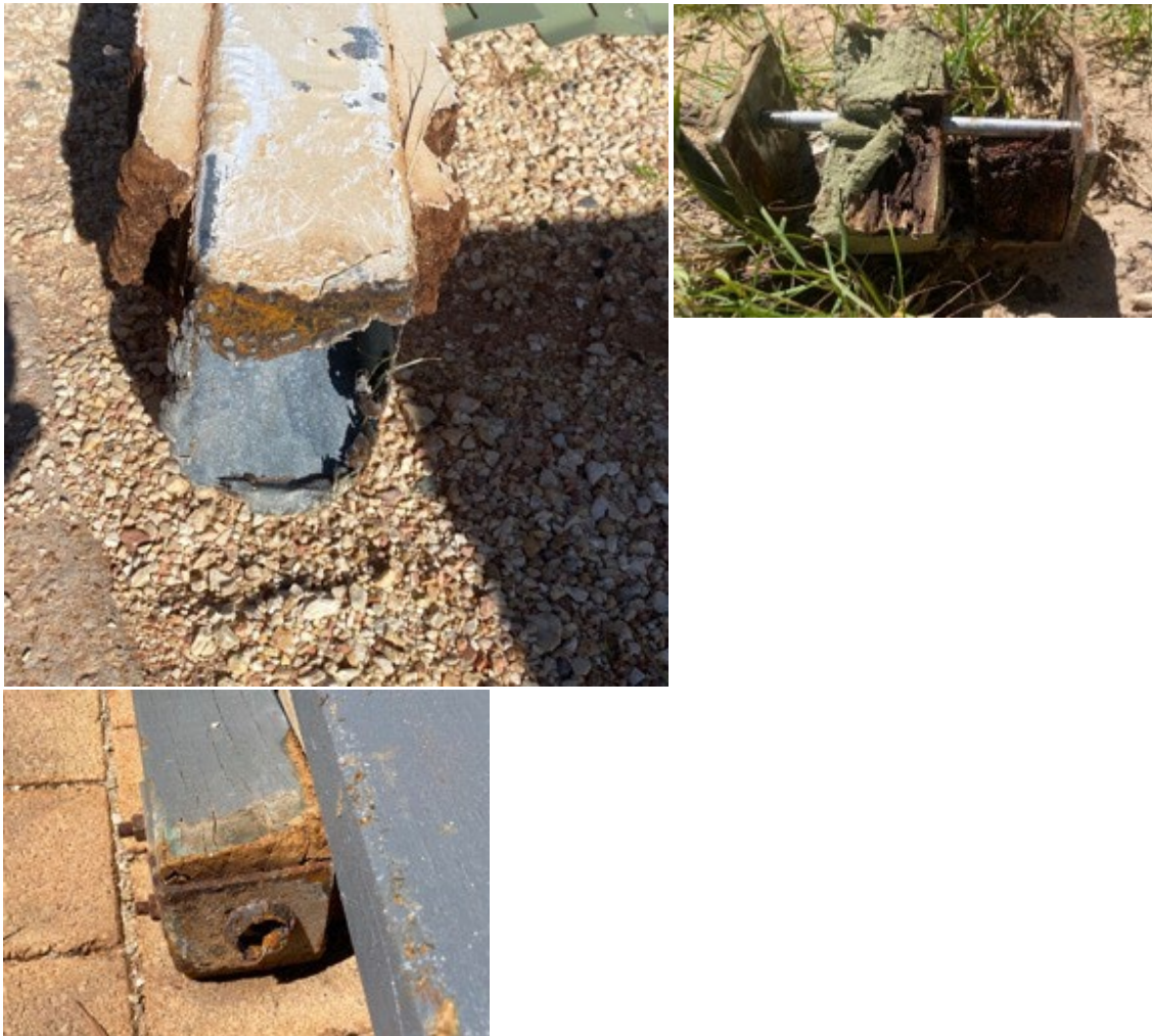
Deterioration of veranda posts at ground line that led to veranda loss
