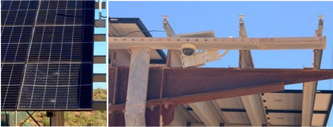
Failure of ground-mounted solar panels, by failure of the glass and loosening of clamps
