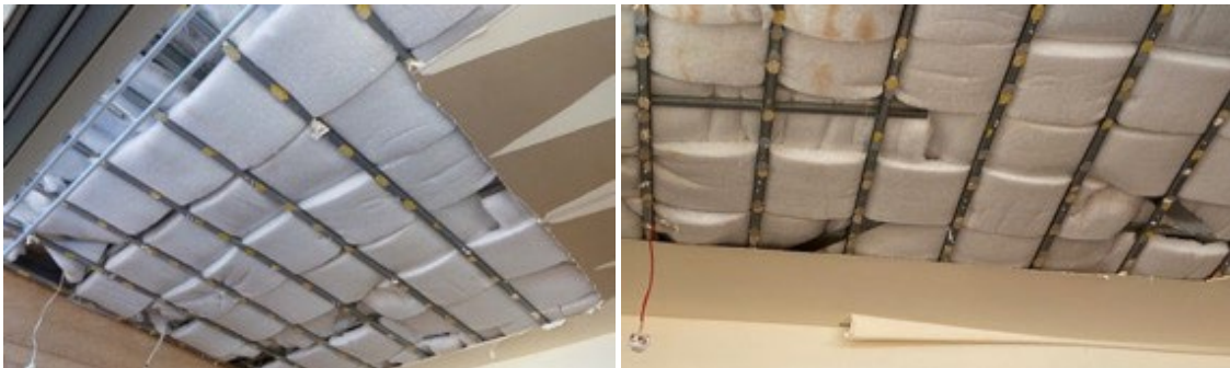
Ceiling loss behind ineffective apron flashing
